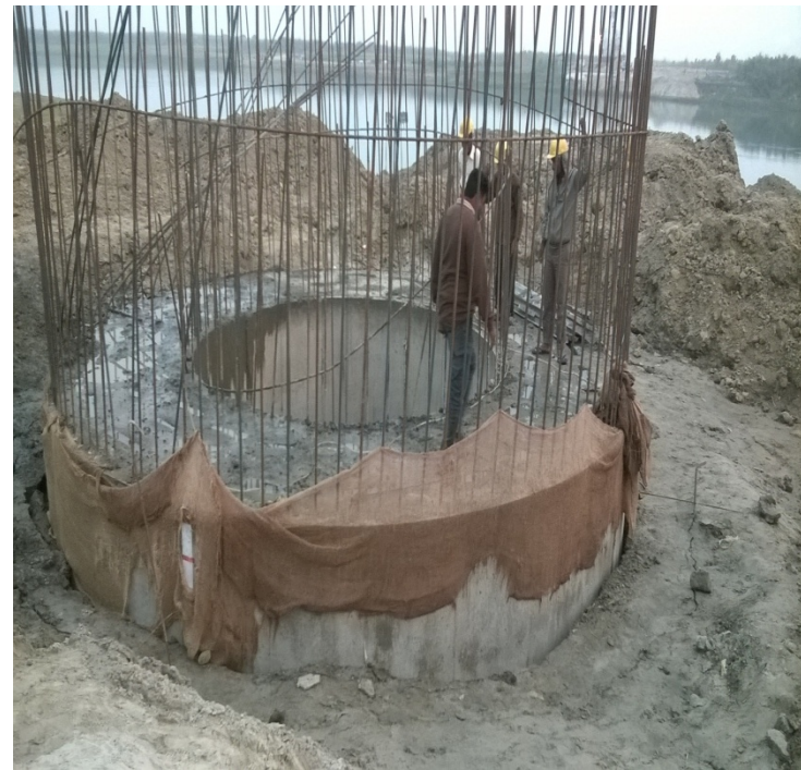
Figure 7- Sand Blow Condition around the well Steining
